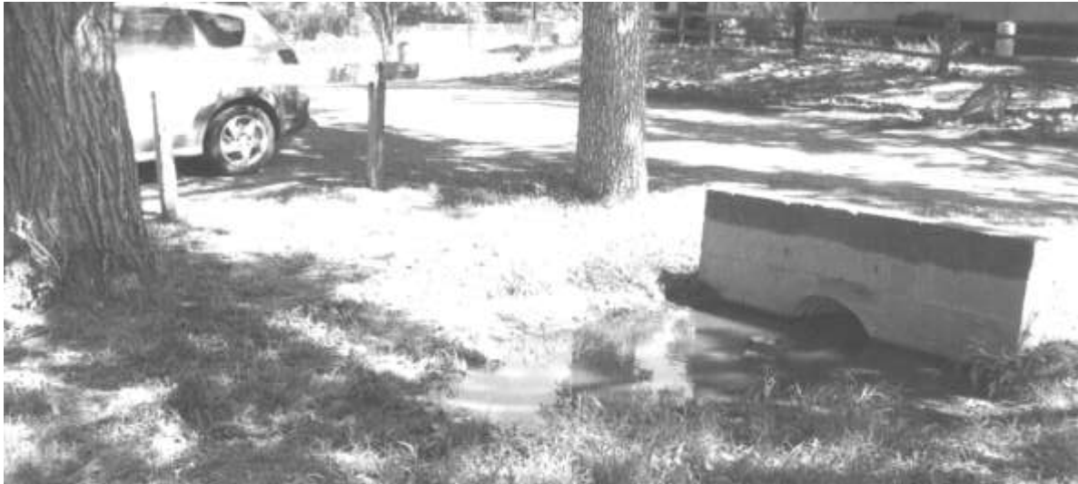
Photograph of the standing water area at the base of the culvert on Quiroga Avenue
